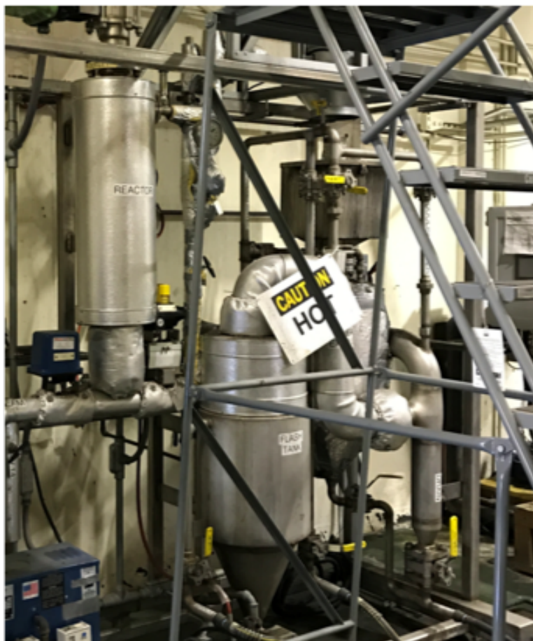
Figure 2.9: The picture of thermal hydrolysis process.
