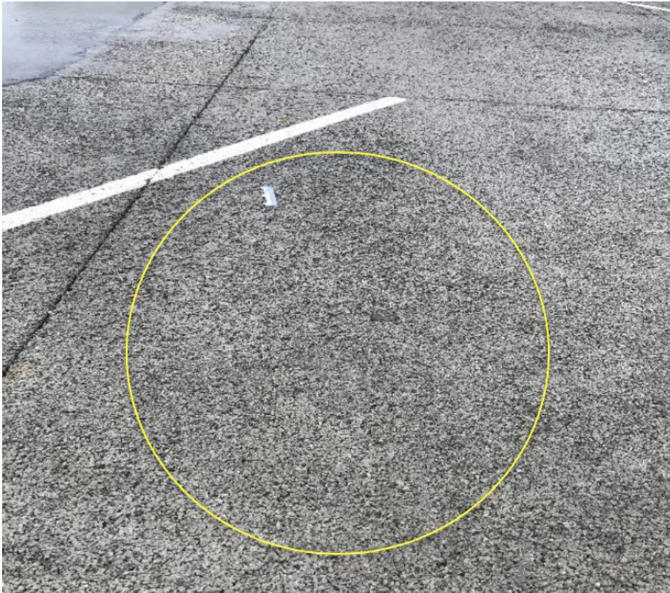
a) Raveling of Surface
