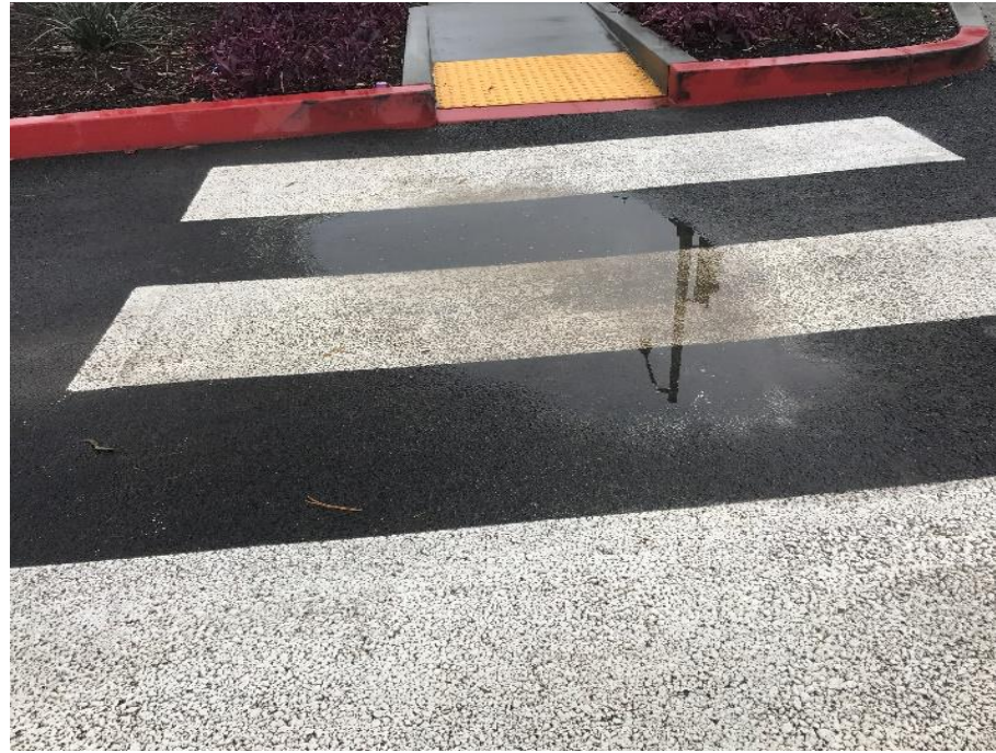
b) Stagnation of Stormwater
