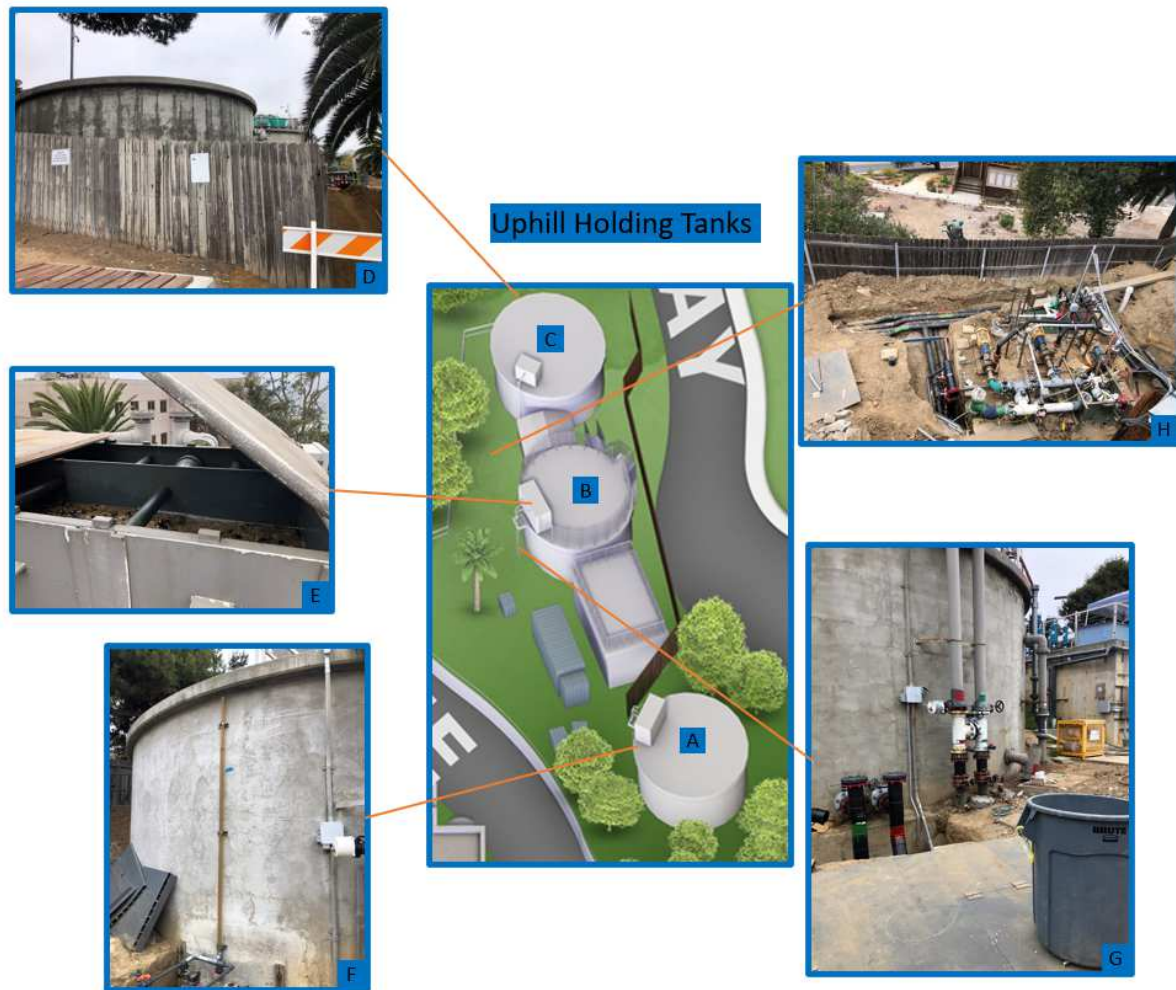
Figure 6: Uphill holding tanks at Pump Station 3. (A) Holding tank #1. (B) Holding tank #2. (C) Holding tank #3. (D) Side view of holding tank #3. (E) Degassers located on top of the tanks. (F) Water level marker (site glass). (G) Dual seawater intake and output lines. (H) Series of pumps and piping serving the holding tanks.
