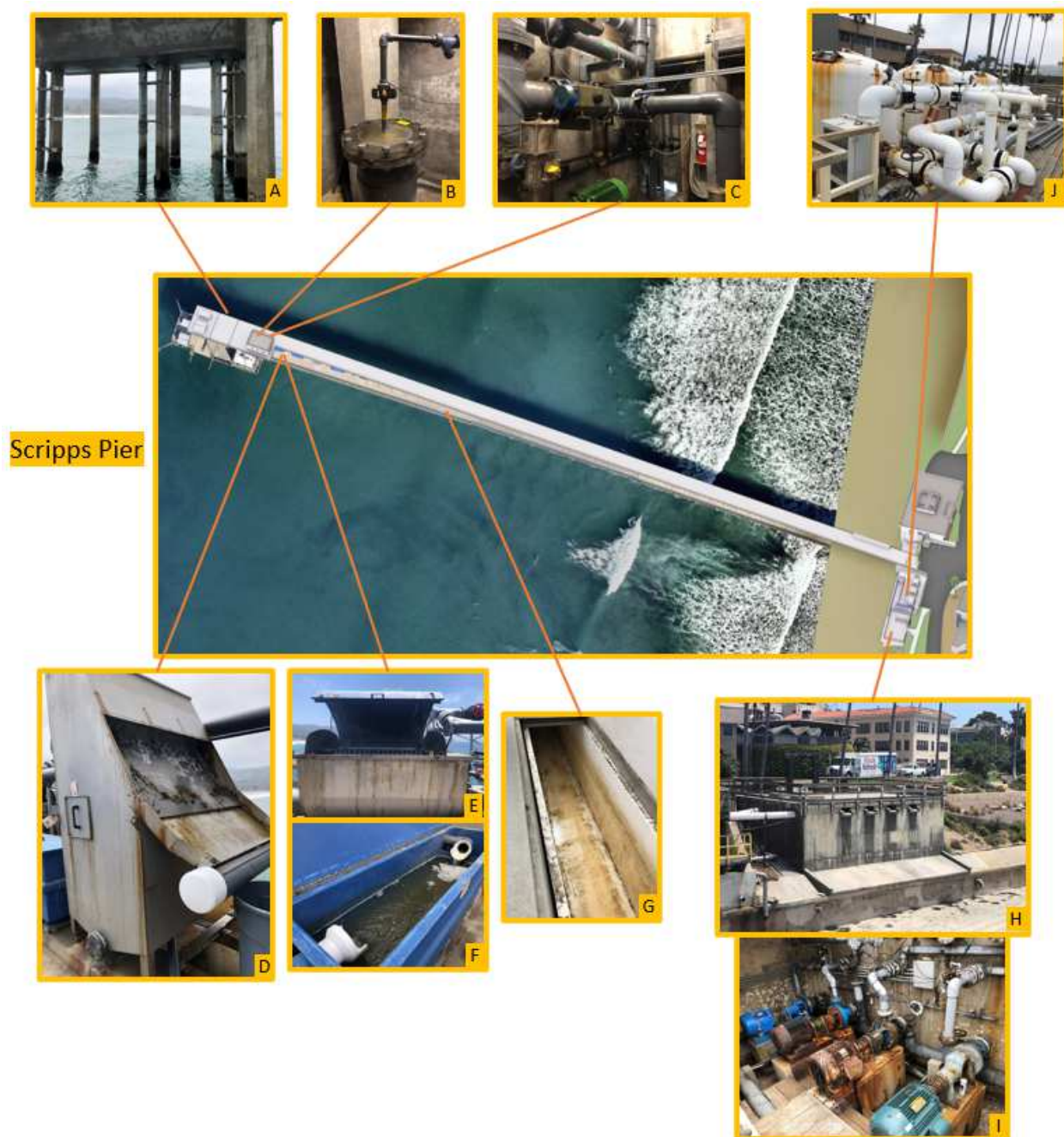
Figure 5: Scripps Pier area (Pump Stations 1 and 2). (A) Seawater inlet pipes at the end of the pier. (B) Inlet pipe connected to vacuum pump line. (C) Water piping inside the pump room. (D) Parabolic screen that newly collected water passes through. (E) Rotating drum filter. (F) Sediment settling tank. (G) Flume used to transport seawater uphill the pier. (H) Seawater settling tanks at base of pier. (I) Pumps used to transport seawater uphill to the holding tanks. (J) Sand filters at base of pier.
