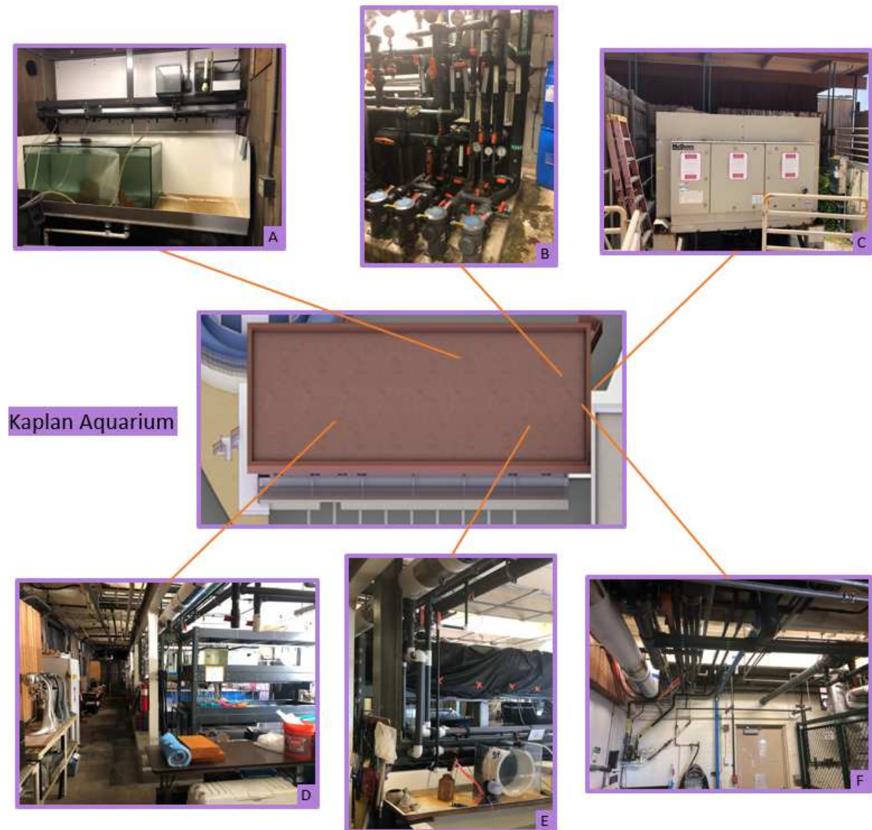
Figure 7: Kaplan Aquarium. (A) Contents of side rooms in Kaplan (B) Heat exchangers and filters. (C) McQuay water chiller. (D) Kaplan interior showing modular racks and seawater plumbing. (E) Example of piping output into a tank. (F) Seawater piping entering the building. The dark gray piping represents ambient seawater and the white piping carries chilled seawater.
