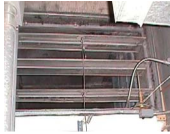
Figure E.4. Exhaust Air Dampers
