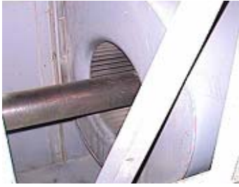
Figure E.3. Air Handling Unit
