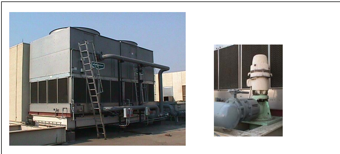
Figure E.1. Cooling Tower
