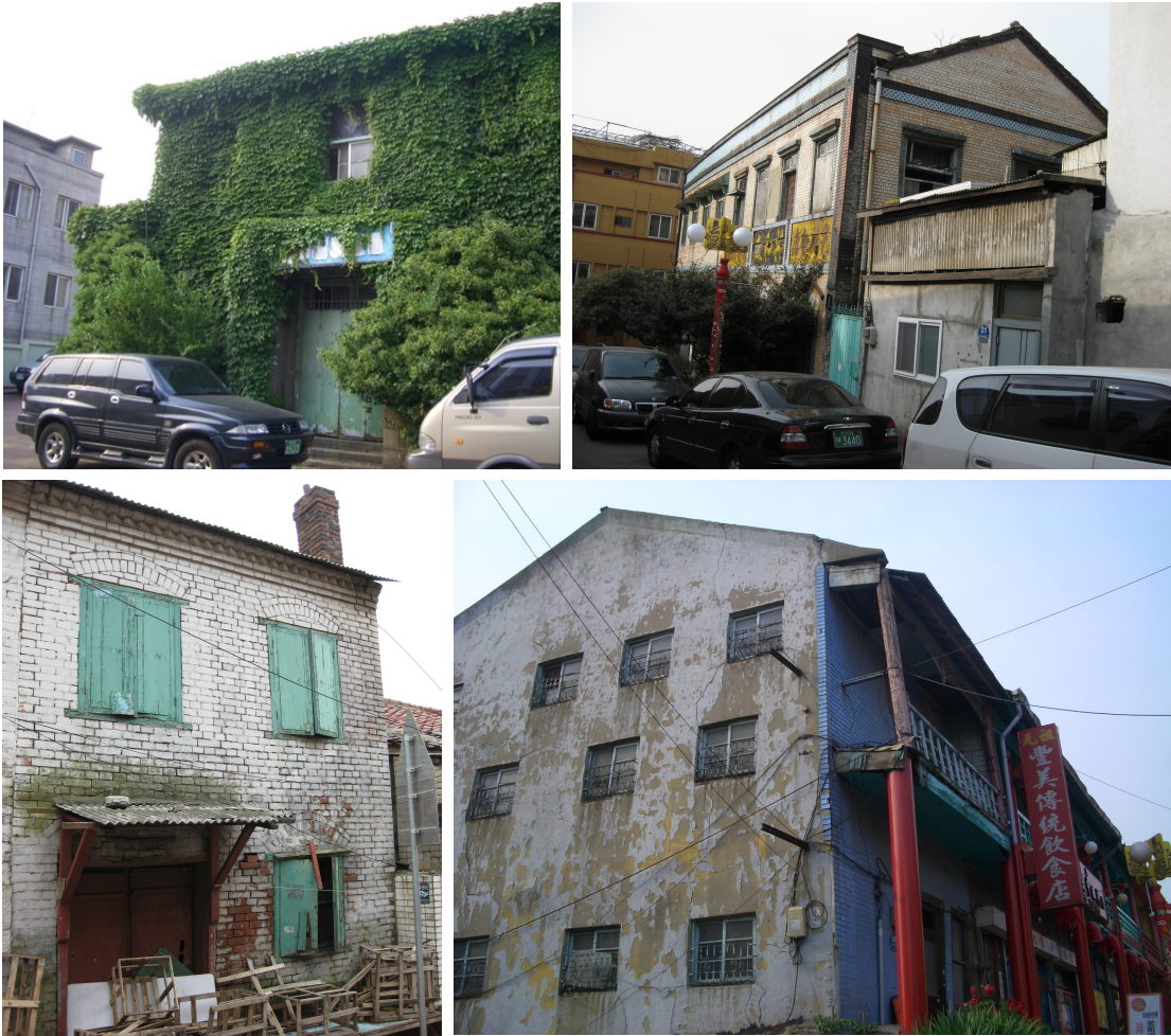
Figure 4-7. Buildings had long stood in neglect, with ivy creeping up or paint flaking off the walls. (Photograph by Sujin Eom (2006-2009))
