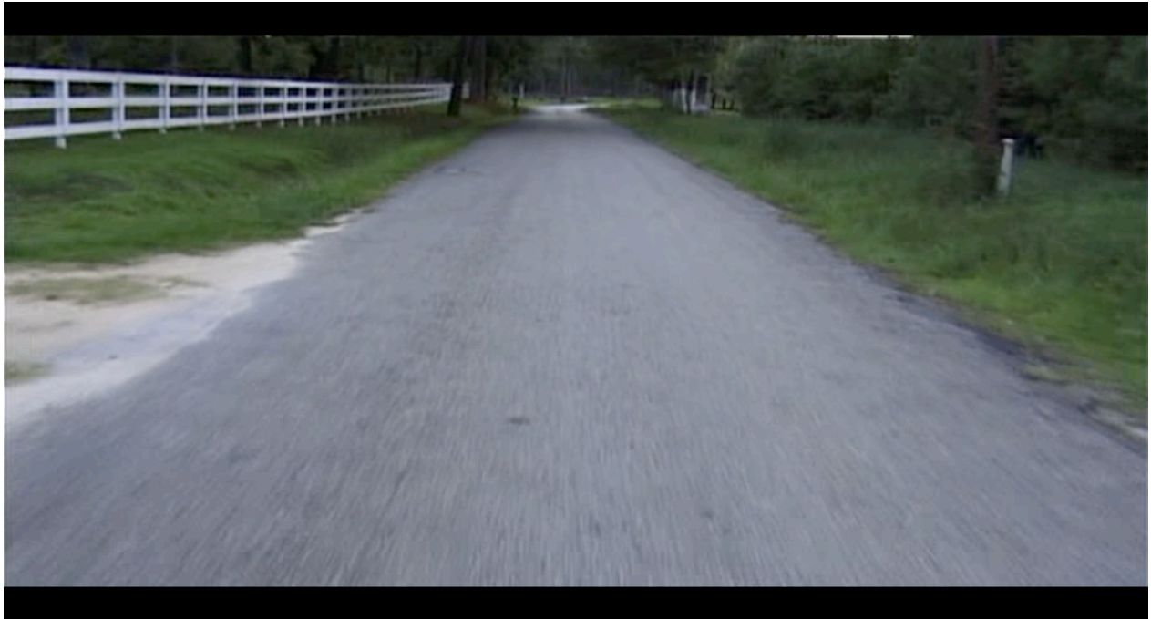
Figure 33: Even the potholes ( Sud )
