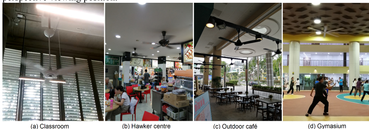
Figure 1. Examples of visual flicker caused when the artificial light installations are placed above the mounting height of the ceiling fan. From certain viewing positions as seen in: (a) classroom, (b) Hawker (food court) centre, (c) outdoor café and (d) gymnasium, the fan blades will obstruct the illuminated area of the light fixture and causes visual flicker.
