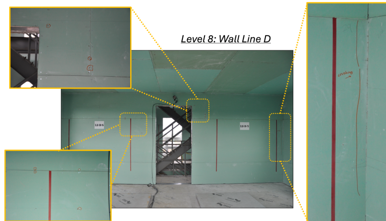
Figure 3. Damage documented post- MID16 , along wall line D at Level 8.
