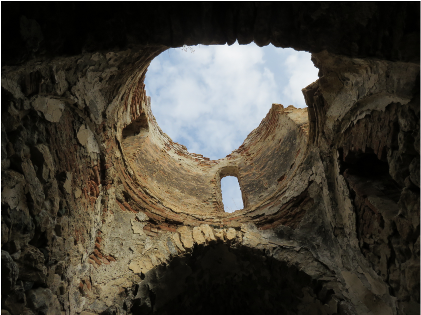
Figure 3.4. The partially collapsed dome of the church of the Holy Mother of God within Der Meryem Monastery. November 8, 2015.
