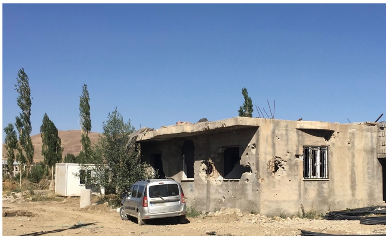
Figure 6.11. A home that was partially destroyed during the curfew in Yüksekova. August 11, 2018.
