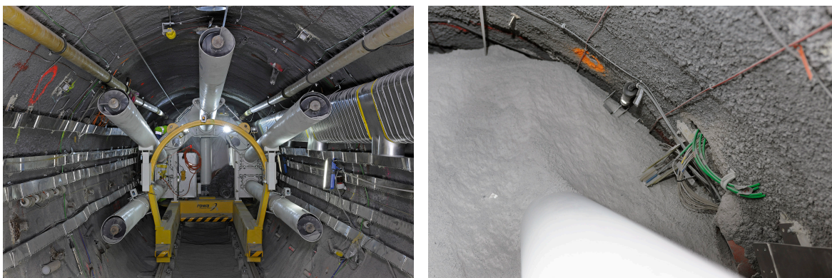
Figure 21–8. Left—The backfilling machine in the FE tunnel. Right—A detail of the emplaced granular bentonite and the contact with the liner.
