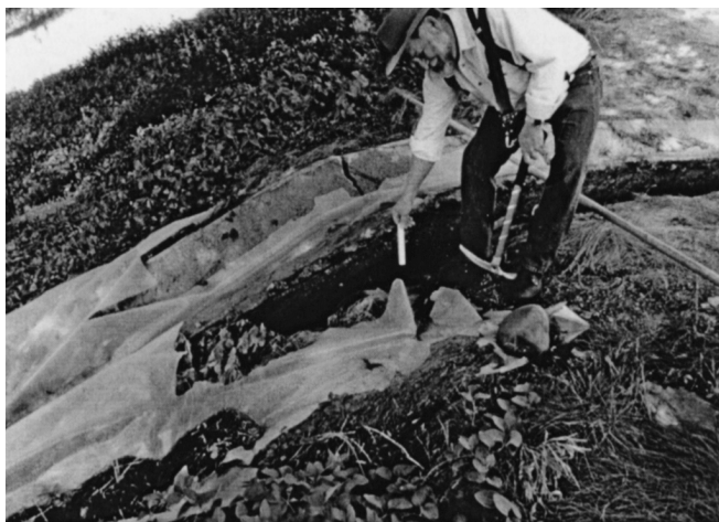
FIG. 8. Uplifted Down Drain Indicating Compression of Fill Slope Face
