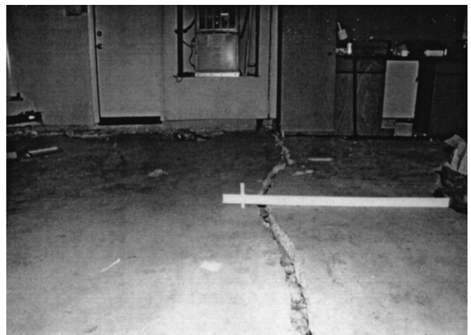
FIG. 5. Cracked Floor Slab above Cut/Fill Contact—Displacements Are 1.9 cm (V) and 5 cm (H)
