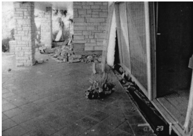
FIG. 7. Evidence of Extensional Ground Deformation at Back of House (Top of Slope Is to Left)
