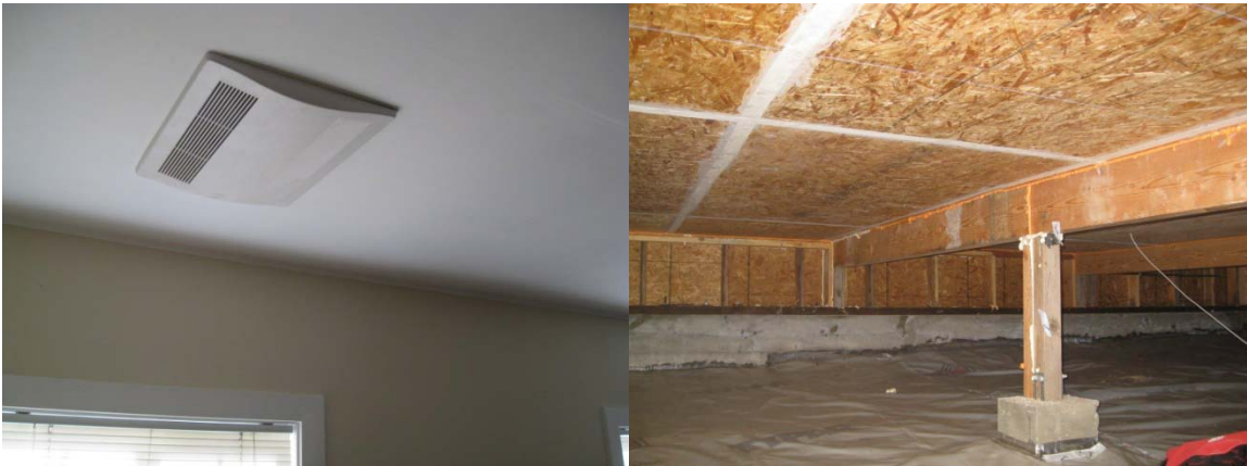
Figure 20 Left : whole house mechanical ventilation was provided by a point-source energy recovery ventilator located in the living room. No distribution was provided to other areas of the home. Right : the unvented crawlspace of the home was air sealed, insulated and water managed.
