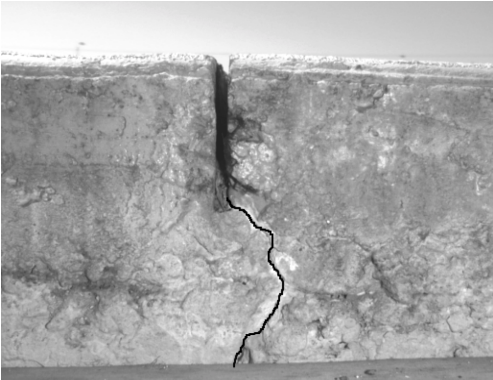
Figure 47b: Photo of Joint 2. Joint crack is enhanced for easier viewing.
