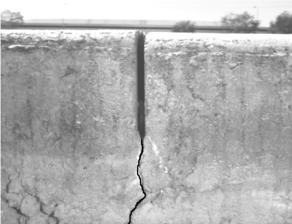
Figure 47a: Photo of Joint 1. Joint crack is enhanced for easier viewing.
