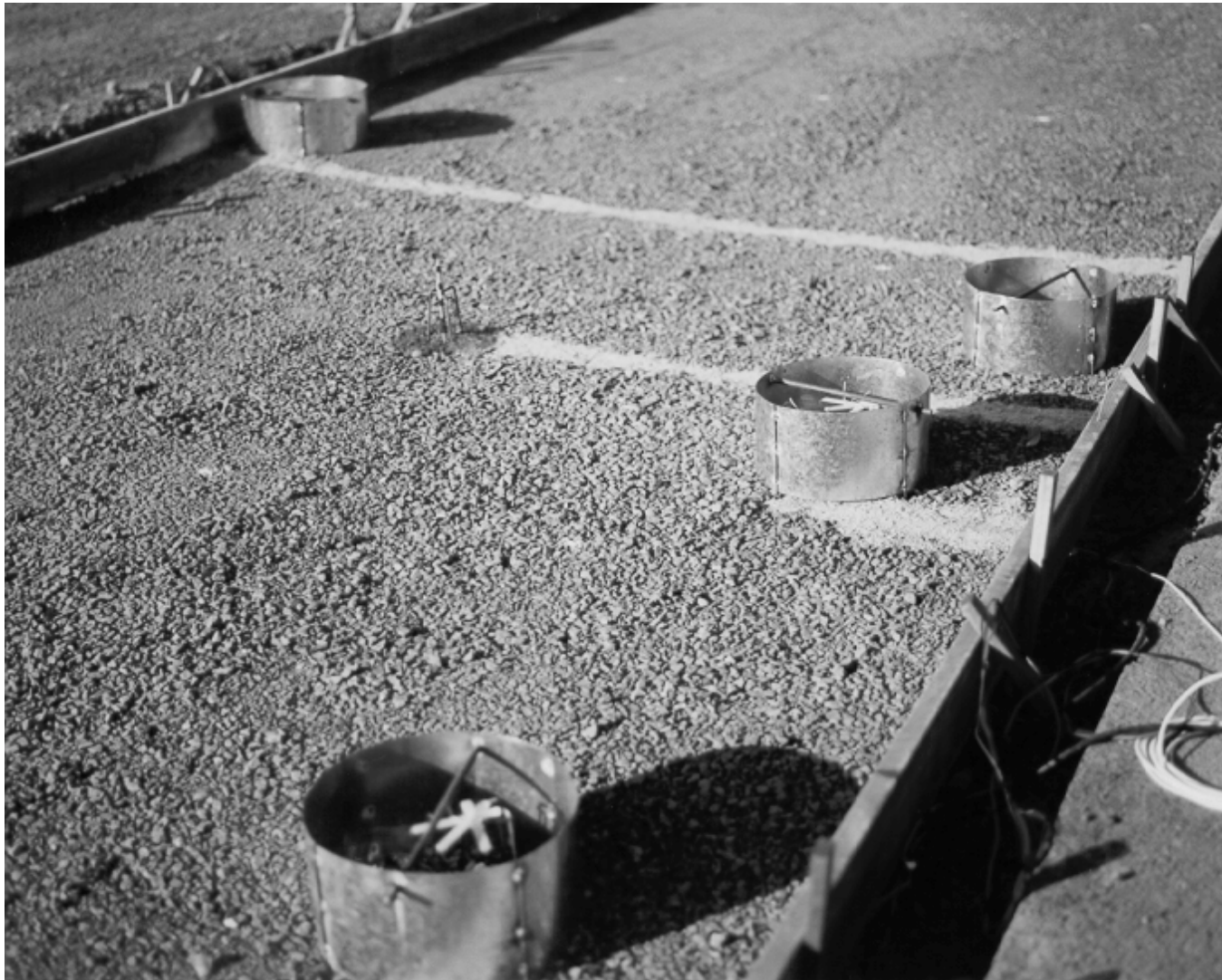
Figure 22. Sheet metal boxes are used to protect strain gages from flow of fresh concrete.
