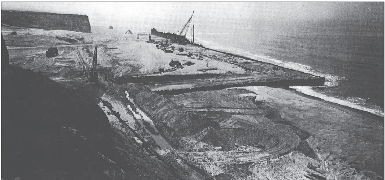
Figure 8. Photo taken 24 June 1964 from Station A showing sand spoil from continued cliff excavation and most of the Unit 1 sheet-pile laydown pad completed.
