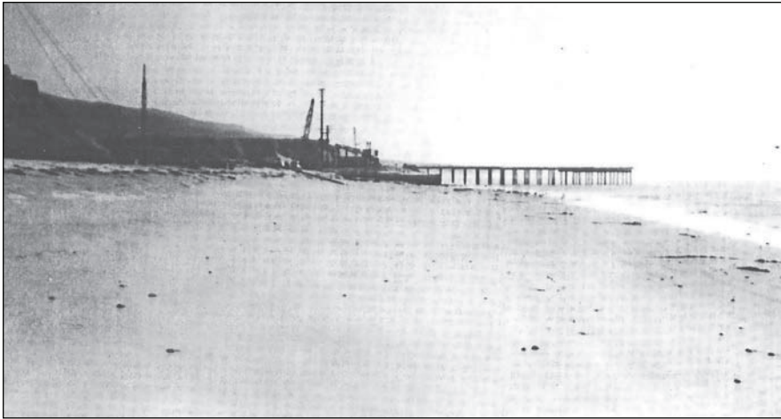
Figure 9. Photo taken 30 January 1965 looking south toward Unit 1 laydown pad and the beginning of construction of the trestle used to lay the cooling pipes.
