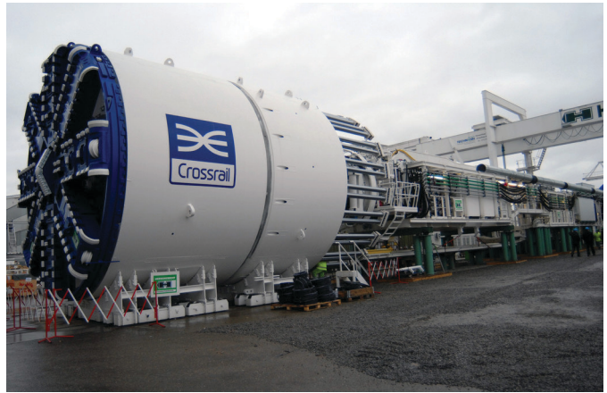
FIG. 1: One of the first of six Crossrail boring machines; each one has its own name: Ada, Phyllis, Mary, Victoria, Elizabeth and Sophia. PHOTO: CROSSRAIL.
