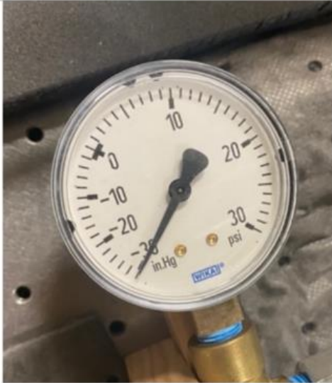
Figure 17: Pressure Gauge from Vacuum Lines
