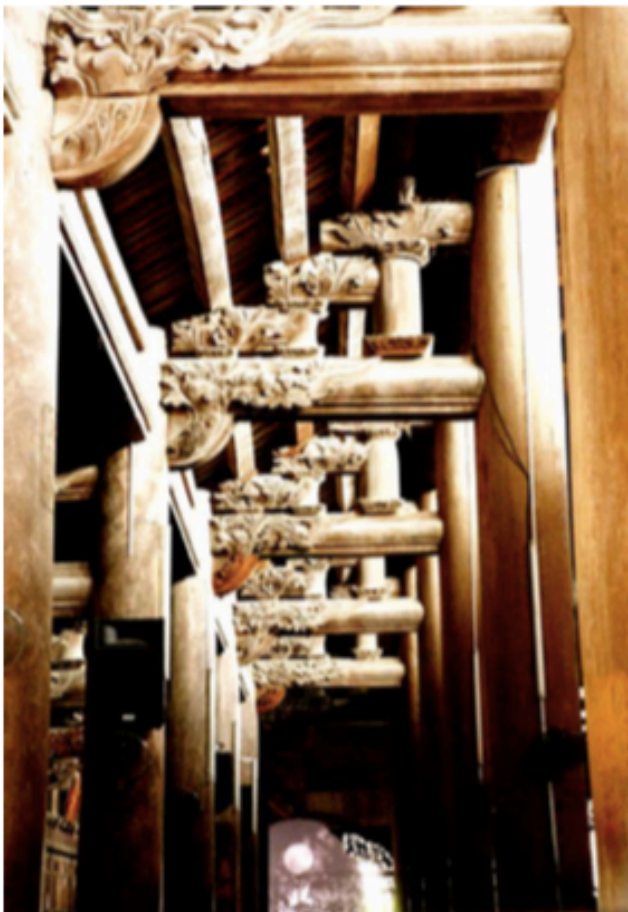
Figure 23. Detail of the cross beams above the aisles, interior of Phat Diem Cathedral, Vietnam.
