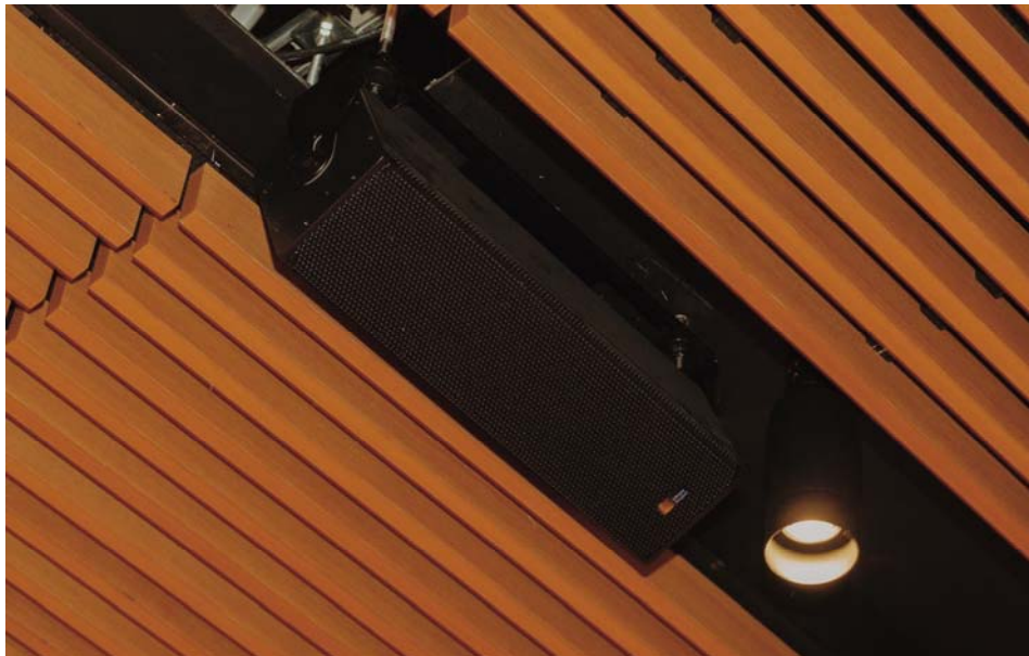
Figure 15: View of Meyer Sound Laboratories UP-4slim Loudspeaker installed in ceiling Photo Credit: H. Scott Roth
