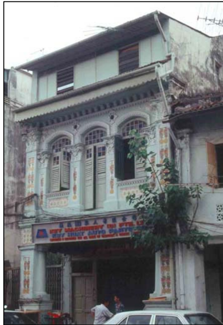
PLATE 3. Deteriorated Shophouses in Niucheshui
