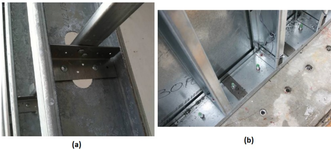
Figure 6.10: (a) Clip placed at utility hole [36] (b) Blast washer and L-shaped bracket installation [22]
