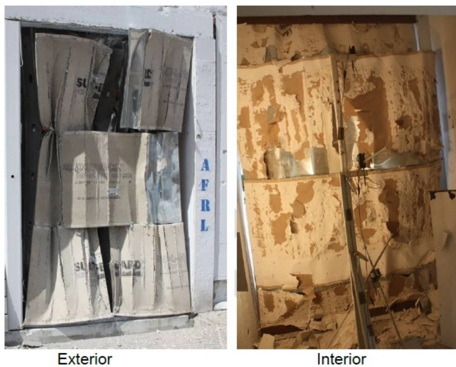
Figure 6.71: Significant exterior panel damage from shockwave [36]
