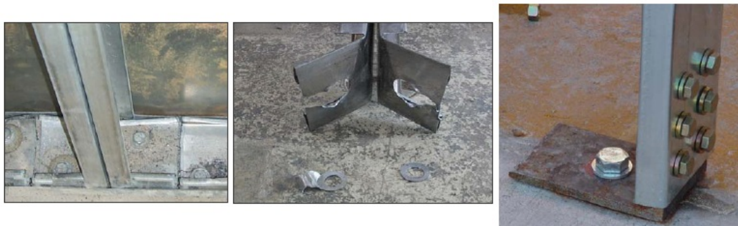
Figure 6.3: Tearing of connection occurs in light gauge sheet [51]
