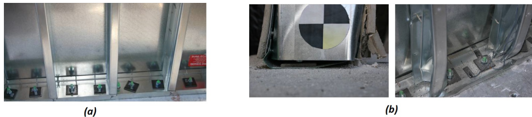
Figure 6.5: (a) Initial series 1 “bearing washer” connection (b) Connection failure mechanism involves warping of track and stud webs [22]
