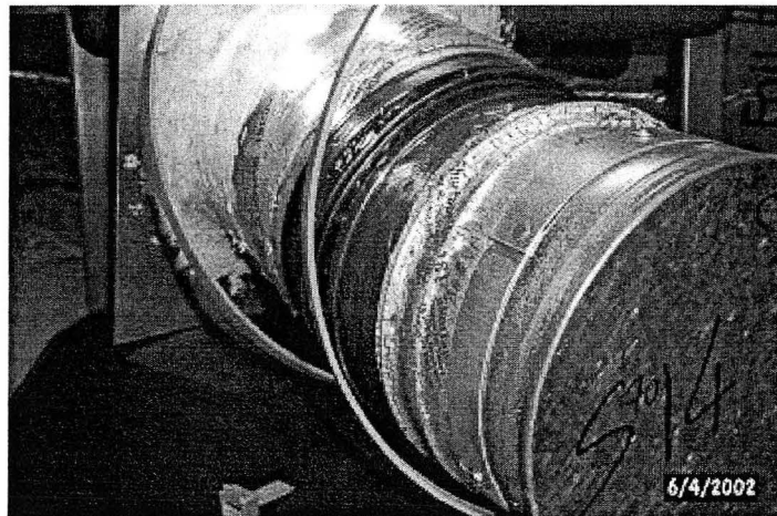
Figure 12. The failed plastic strapping on one of the flexible core to sheet metal collar specimens after four months of aging.
