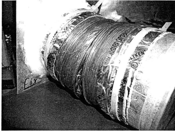
Figure 11. Oozing of the adhesive layer in the foil-butyl tape (Tape 4) specimens (showing result of 5 months of aging).
