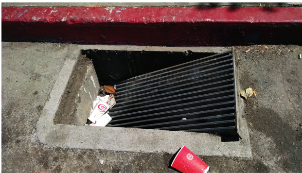
Figure 1. Hole next to the sidewalk.
