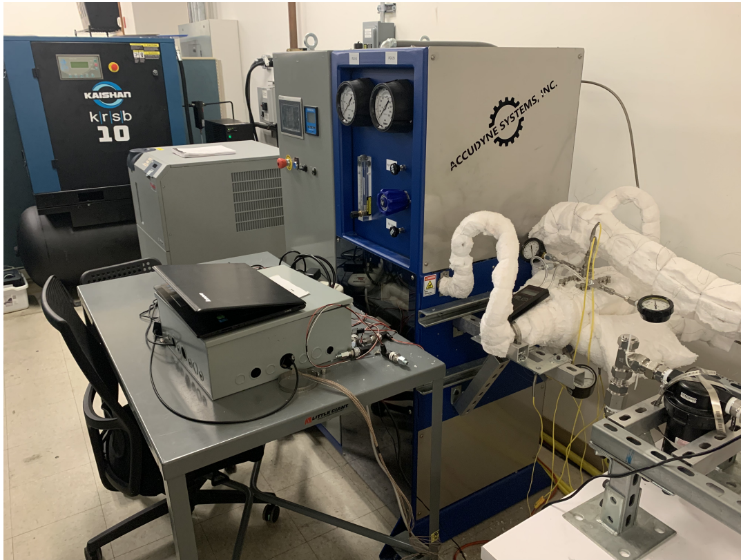
Figure 2.2: sCO 2 experimental system with installed test part.
