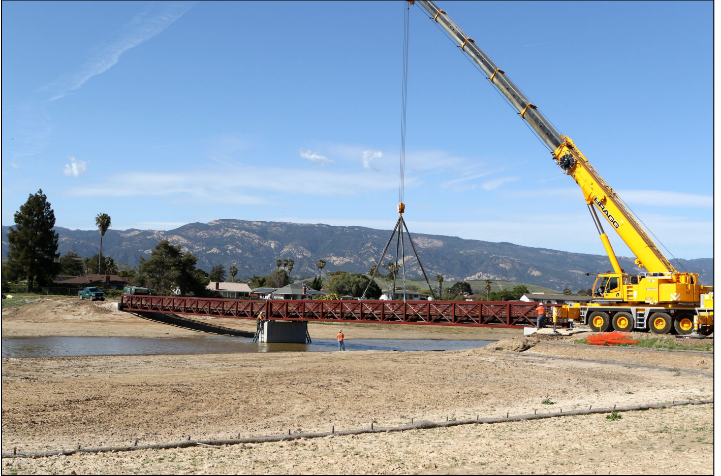
Installation of the main bridge at NCOS on April 18, 2018. Photo courtesy of David Levasheff.
