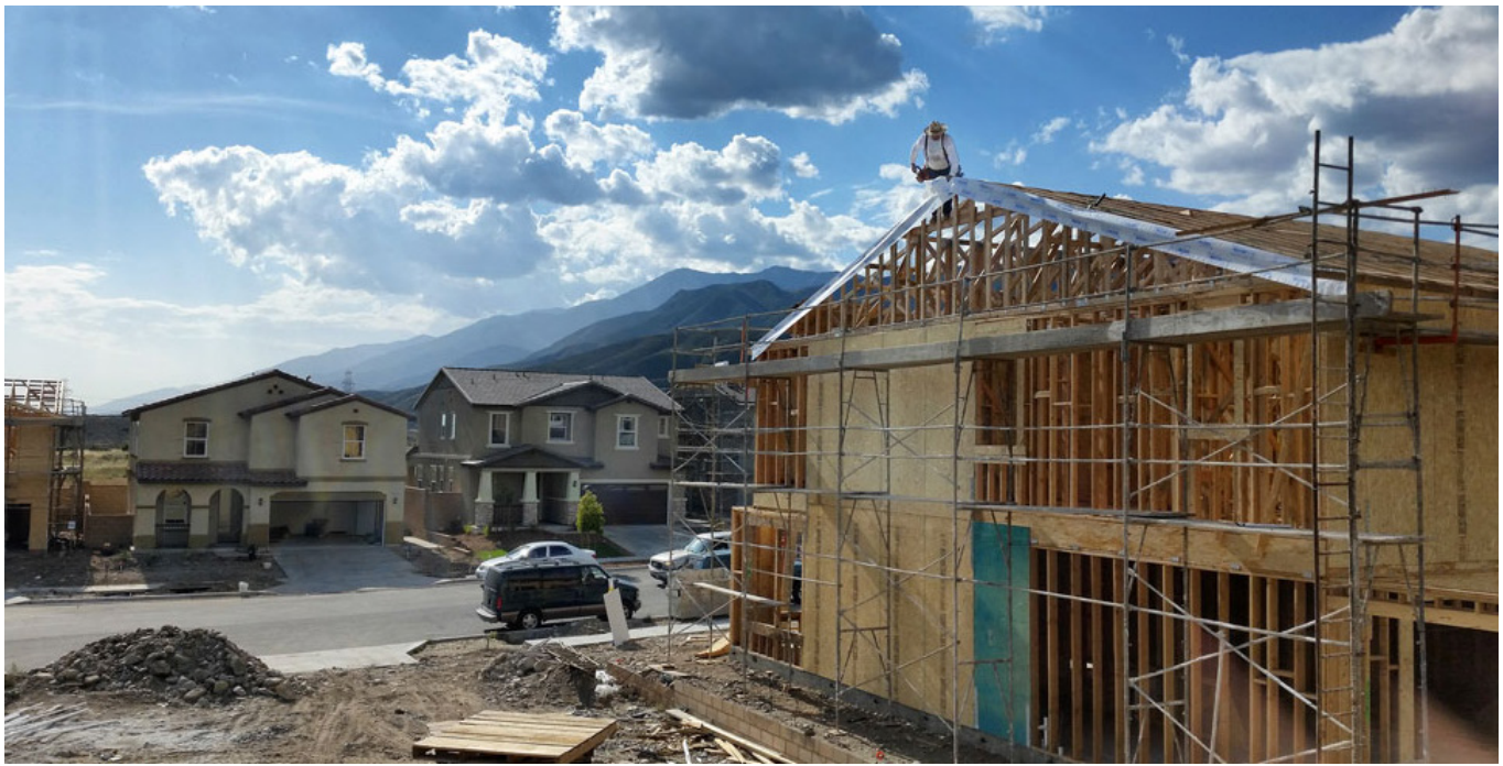
Construction in a suburban neighborhood in Rialto, a small community bordering San Bernardino. Rialto has grown rapidly in past years due in large part to the area's expanding distribution industry. Photograph by Michael Kirk.
