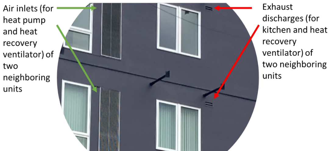
Figure 1. Example layout of exhausts on multi-family residence.
