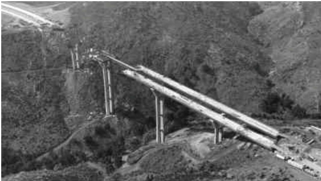
Figure 2-13 Pine River Bridge, San Diego, CA - The First Cast-in-Place Segmental Bridge in the United States (Opened to Traffic 1974)
