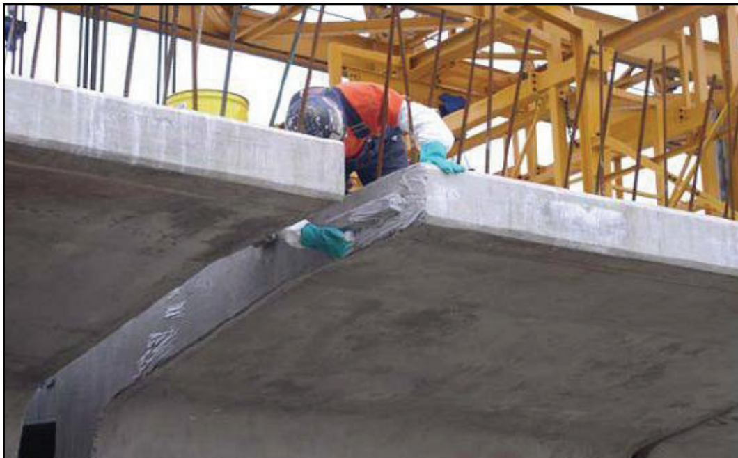
Figure A-13-50 Otay River Bridge - Application of Epoxy to the Segment Joints (Courtesy of International Bridge Technologies)
