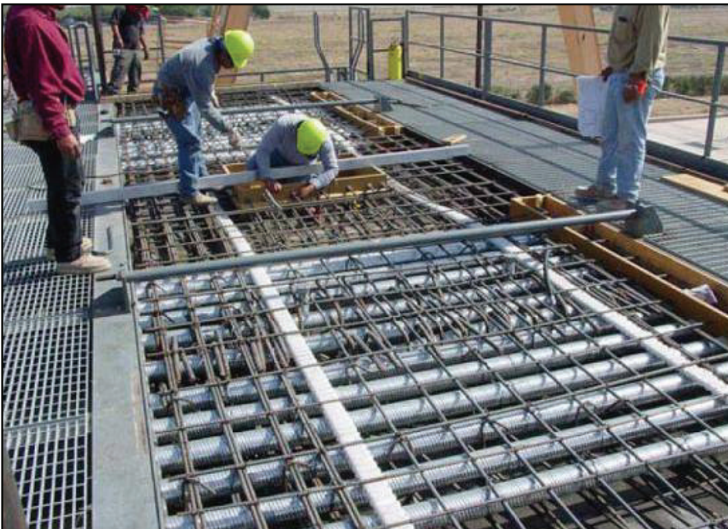
Figure A-13-44 Otay River Bridge - Deck Rebar and PT (Courtesy of International Bridge Technologies)
