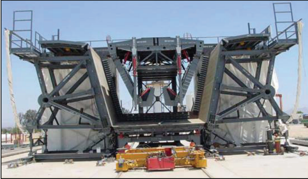
Figure A-13-43 Otay River Bridge - Segment Forms (Courtesy of International Bridge Technologies)
