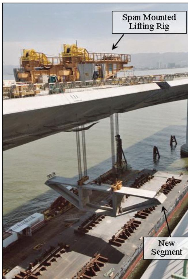
Figure 2-16 Lifting Operation for Balanced Cantilever Construction with Precast Segments and Span Mounted Lifting Equipment
