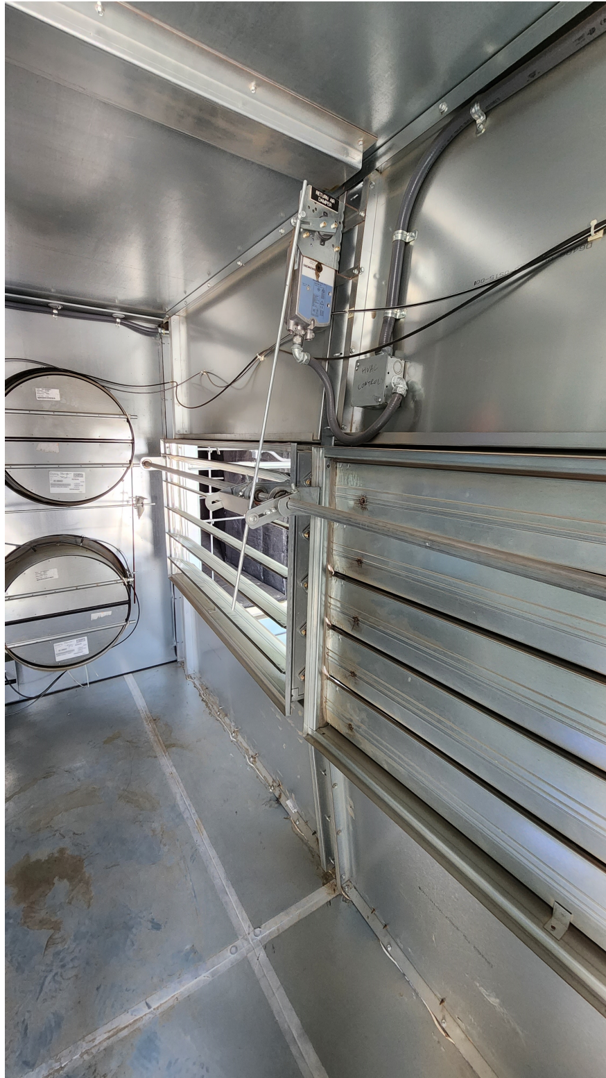
Figure F.1: Damage to TLC AHU1 Plenum
