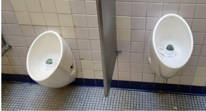
Figure 11: Waterless urinals tested at Dunnigan northbound rest area.
