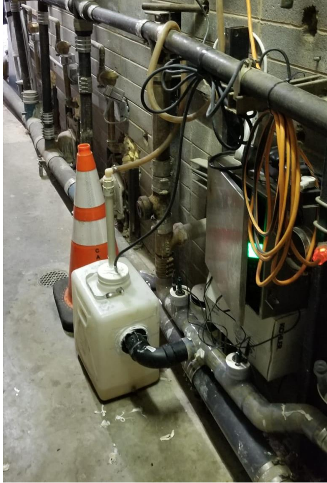
Figure 12: Sedimentation tank in the urine drain line gallery at the Dunnigan northbound rest area.
