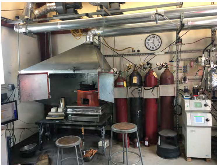
Figure 5.4: Testing setup of BIS under steel exhaust hood at LBNL.
