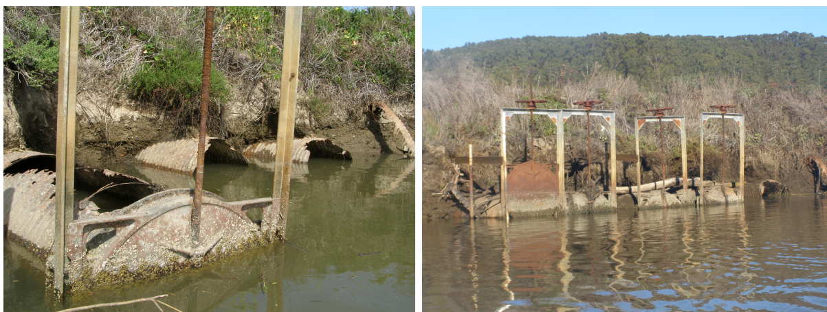
Figure 4.15: Photographs of culverts to North Pond, left photo 23 March, 2010, right photo 29 November, 2010. There has been further deterioration of the culverts since these photographs were taken.
