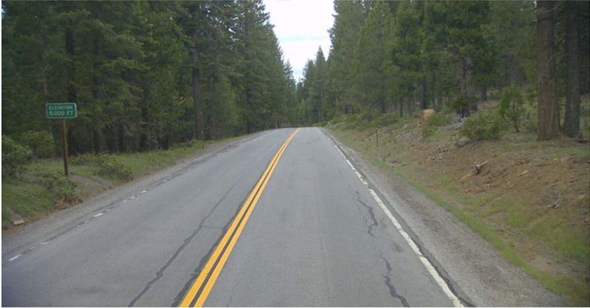
Figure 4.27: Road condition on Sierra 89N PM 28.06 in 2010.
