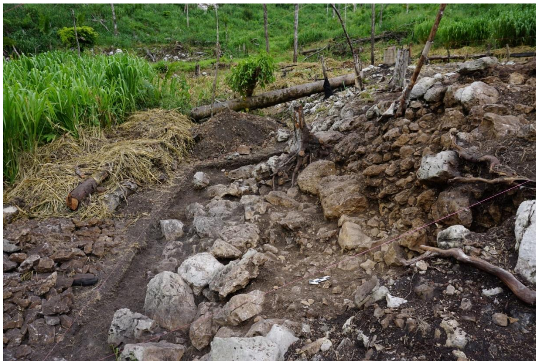
Figure 97. The mound is shored up on the eastern side with a series of boulders, filled in with cobbles and other dry fill material.
