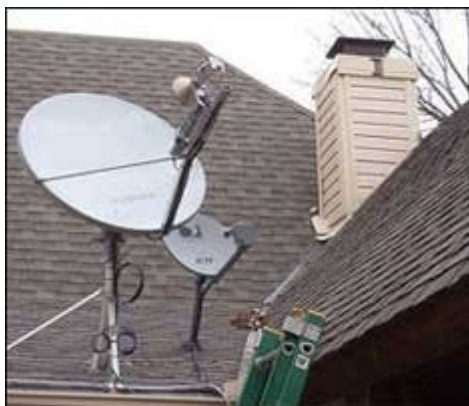
Fig. 1-5. Residential offset reflector Satcom antennas. (Photo from www.reformation.org .)
