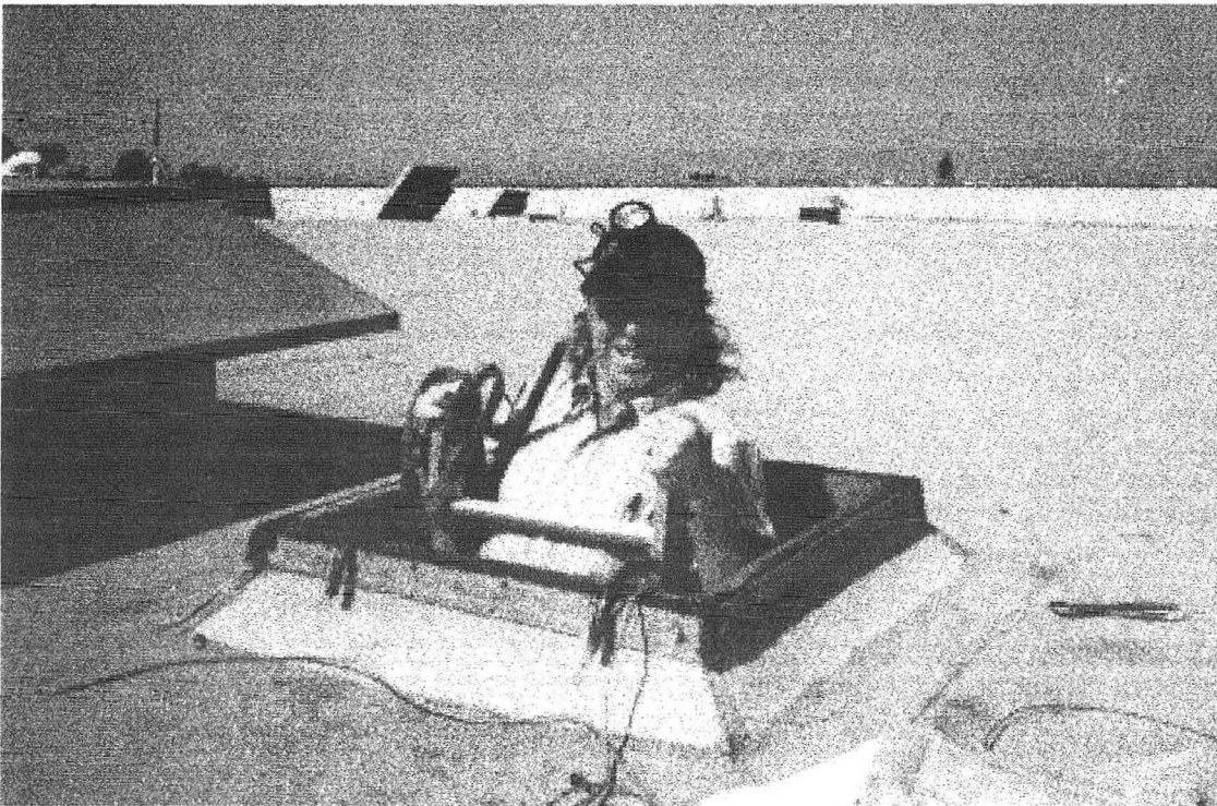
Figure 2.6 Rooftop of Long's Drug Store in San Jose California, tan capsheet with 0.16 solar reflectance.
