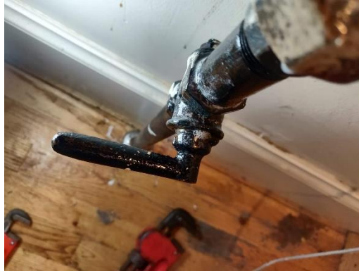
Figure 3.9 A leaky valve identified at Location 1
