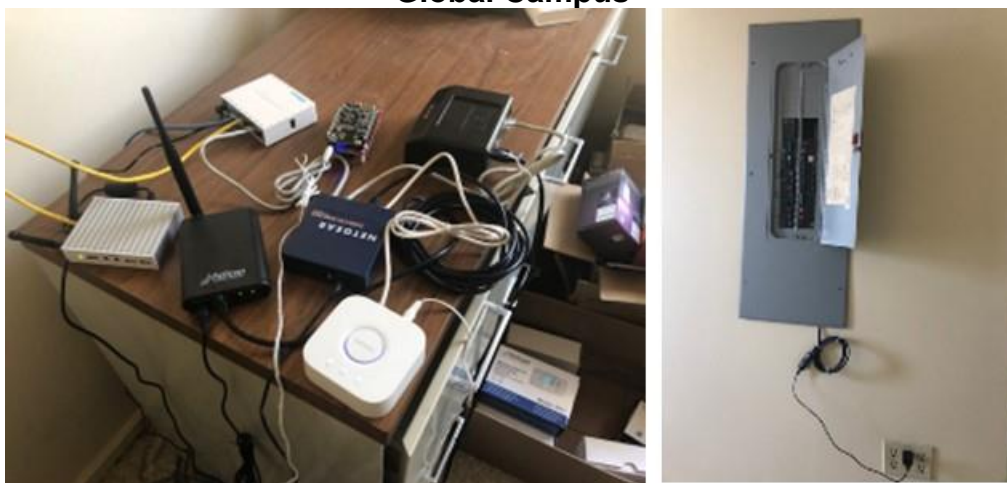
Figure D-2: XBOS-V System (left) and TED Energy Monitor (right) at UC Berkeley Global Campus
