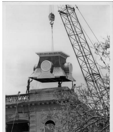
Figure 5 Replacing the turrets during the restoration by the Friends, circa 1960s. Courtesy Hawaii State Archives, Photograph Collection, PP-10-10-030.
