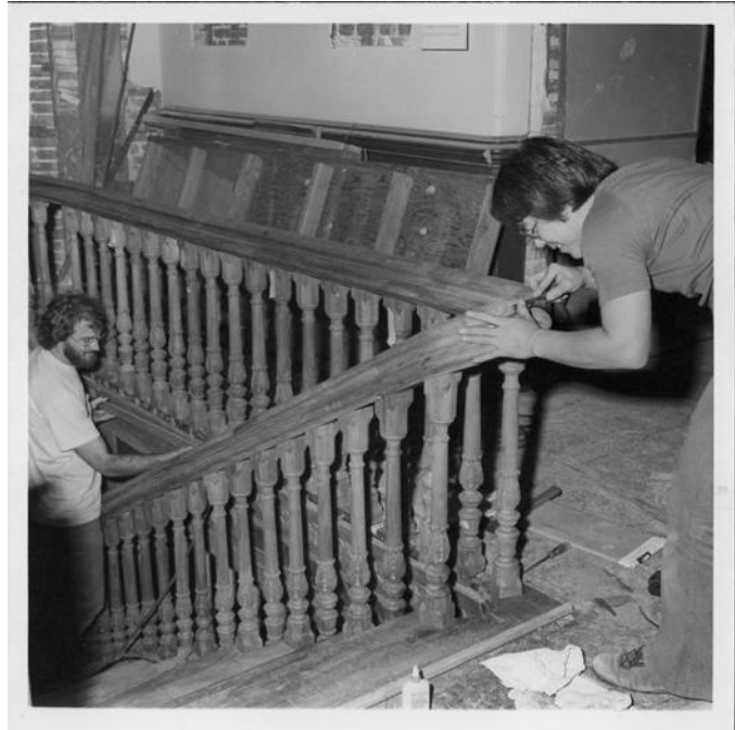
Figure 6 An example of the 1960s restoration work conducted by the Friends of ‘Iolani Palace. Courtesy Hawaii State Archives, Photograph Collection, PP-11-7-023.
