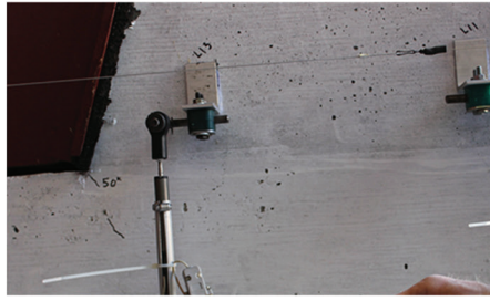
a) Damage Stage I: first diagonal crack observed at 50 kips/222 kN (east face of Shear Key 8A)
