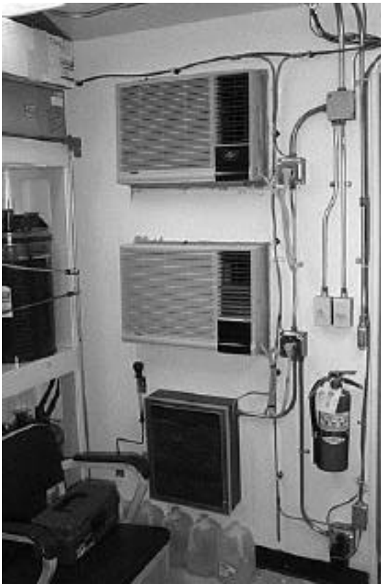
Figure 2: Air-conditioners and Resistance Heater
