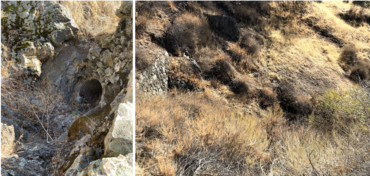
Figure 15: (a) Left: Upstream culvert with pipe (b) Right: Downstream of North Gate Road culvert.
