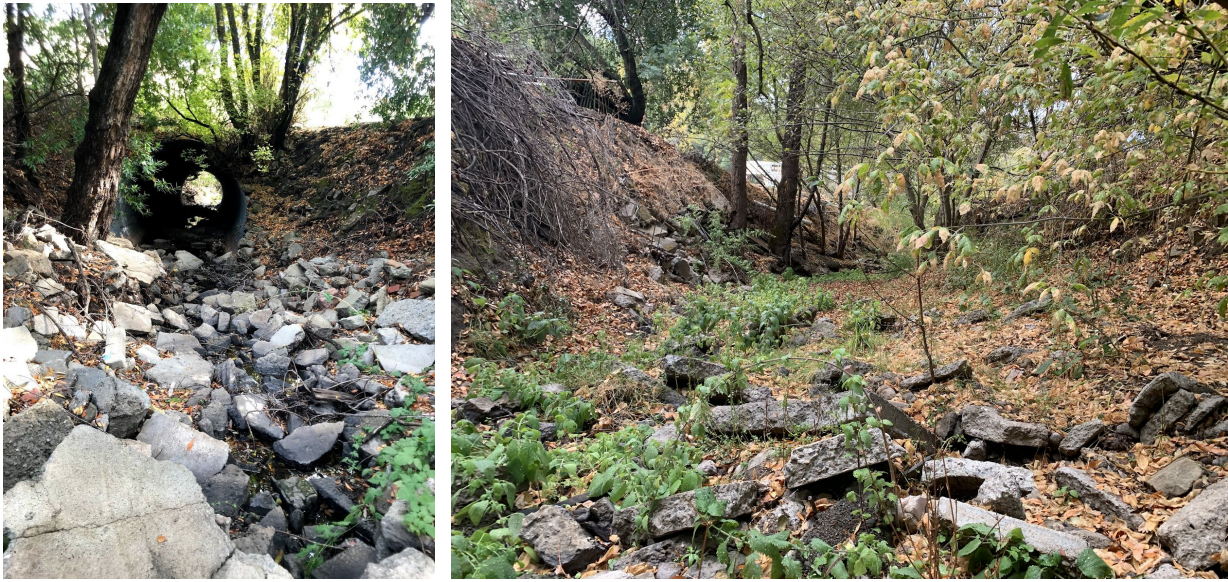
Figure 13: (a) Facing downstream, corrugated metal pipe culvert. (b) Facing upstream with riprap.
