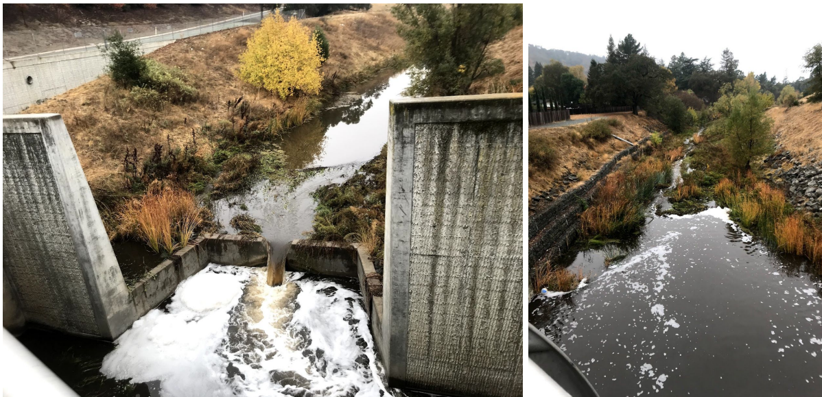
Figure 9: San Ramon Creek at Livorna Rd. (a) Left: Concrete drop structure. (b) Right: Downstream view.
