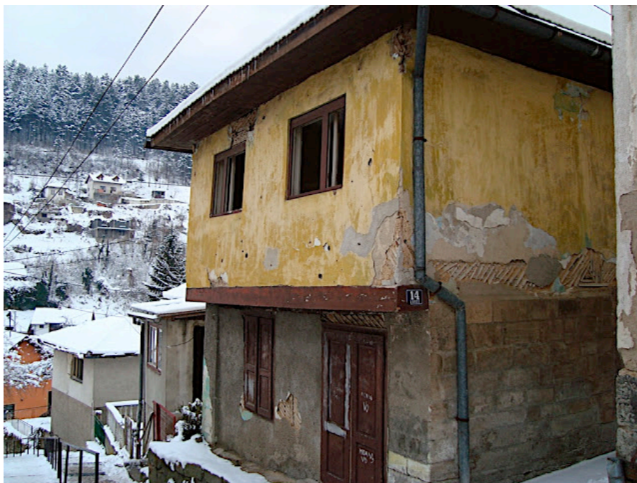
Figure 5: A dilapidated house whose reconstruction has been abandoned.
