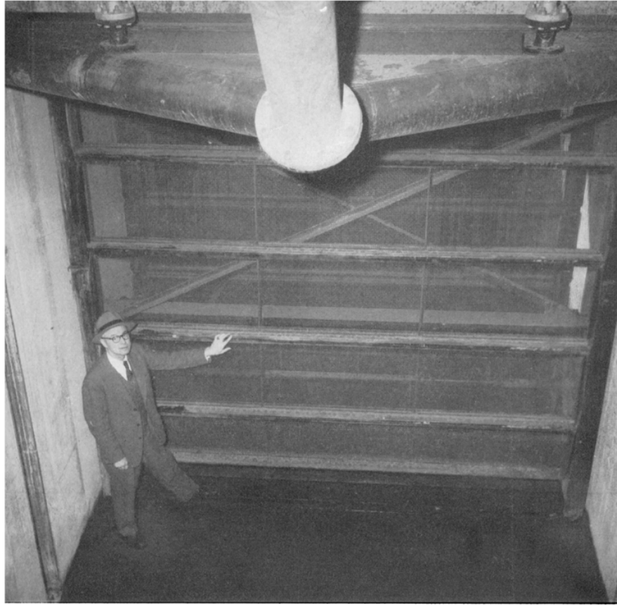
FIGURE 32. Shows fish collector in position in front of traveling Screen 5. Collector extends under curtain wall to within five inches of screen face and the top is open on far side. Photograph by Don Krogh, P. G. & E. News Bureau, March, 1953.
