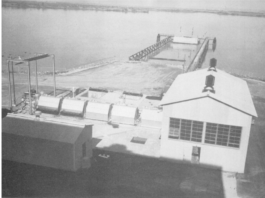
FIGURE 30. Shows screen structure and five traveling screens in the foreground and water intake structure in the river. Building at the right houses cooling water pumps for Units 4 and 5. Tide at time of picture at approximately elevation -2.0 feet. Photograph by Don Krogh, P. G. & E. News Bureau, March, 1953.
