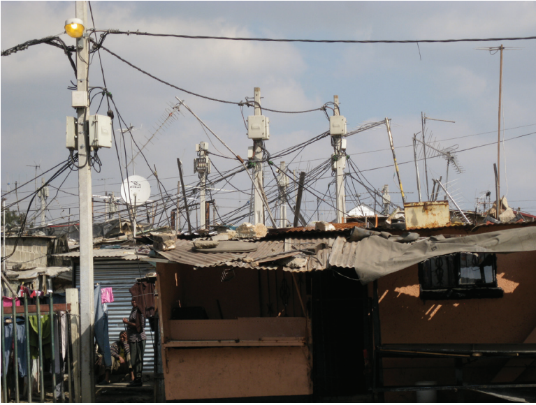
Electric Posts, Township of Alexandra, Johannesburg (South Africa)
