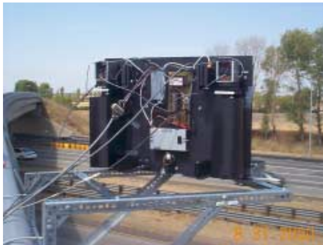
Figure 4.1: Detection System Mounted Above the Highway
