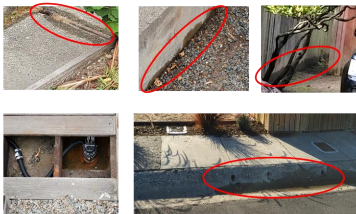
Figure 3.3: Evidence of shallow groundwater in Tamalpais Valley (red ovals, top row) and sump pump, lower left and sump pump discharge pipes (lower right)
