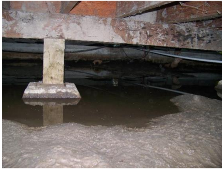
Figure 3.4: Photo of crawlspace water which has been observed in the wet season (photo from Barbara Postel)
