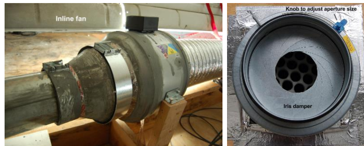
Figure 2. Inline fan and damper used to control air flows
