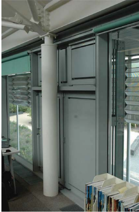
Figure 11: Automated openings for natural ventilation at Heelis National Trust
