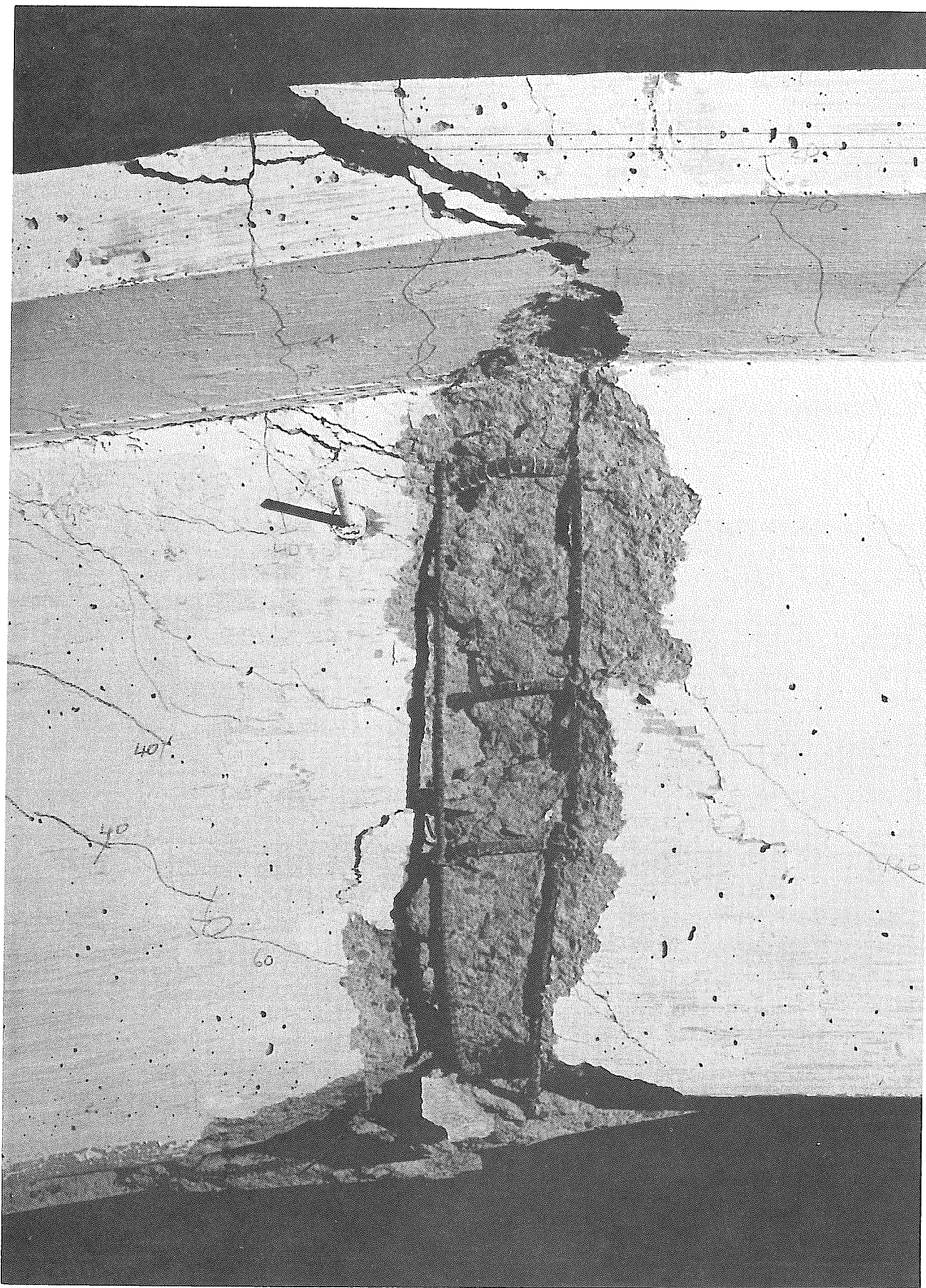
FIG. 81 FAILURE DETAILS AT SECOND HINGE IN GIRDER 1
