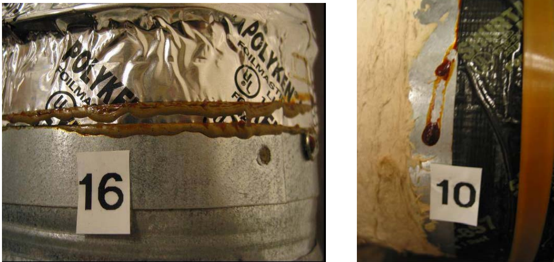
Figure 3. These samples show oozing of the adhesive at the tape edges.
