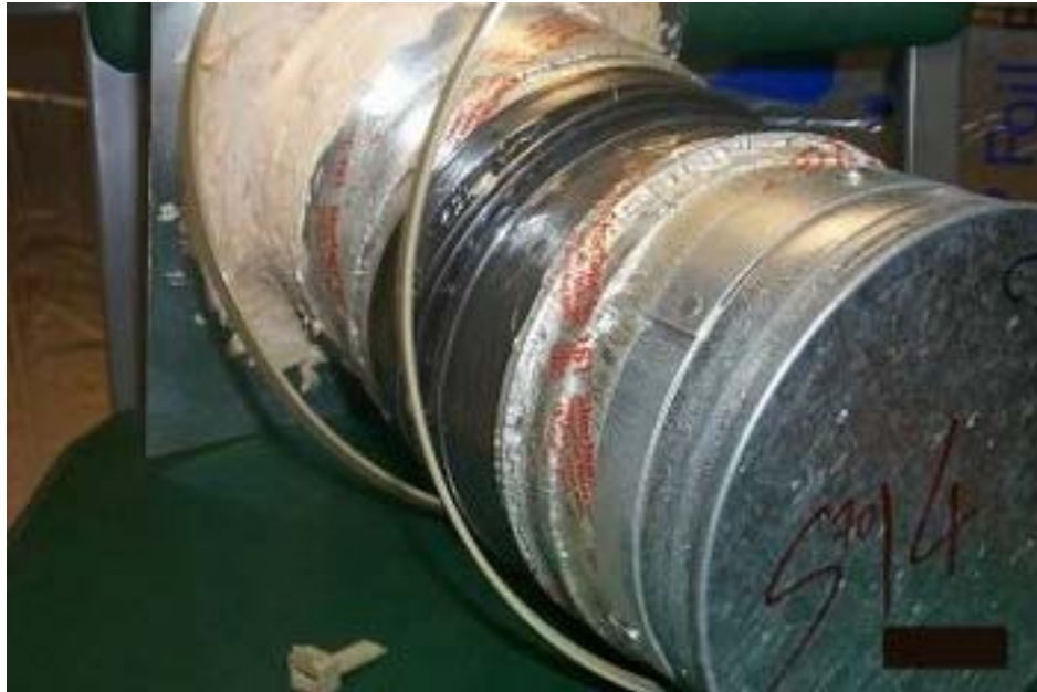
Figure 6. Failed plastic strapping after four months of aging.
